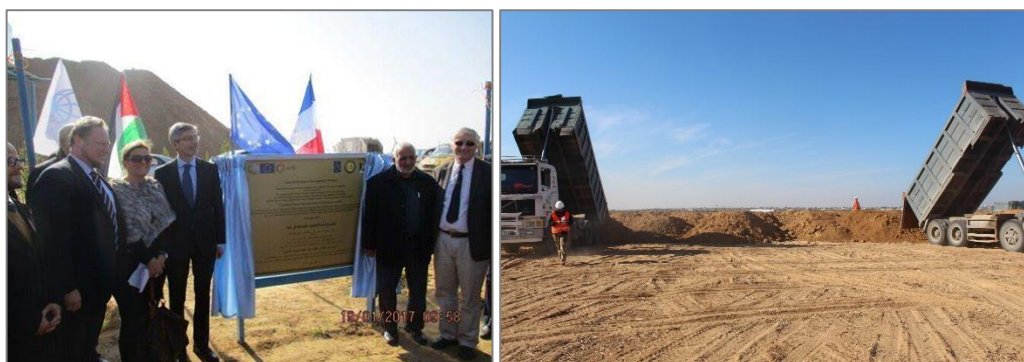
Figure12 . Photos of the excavation work in the new landfill in Al-Fukhary area
