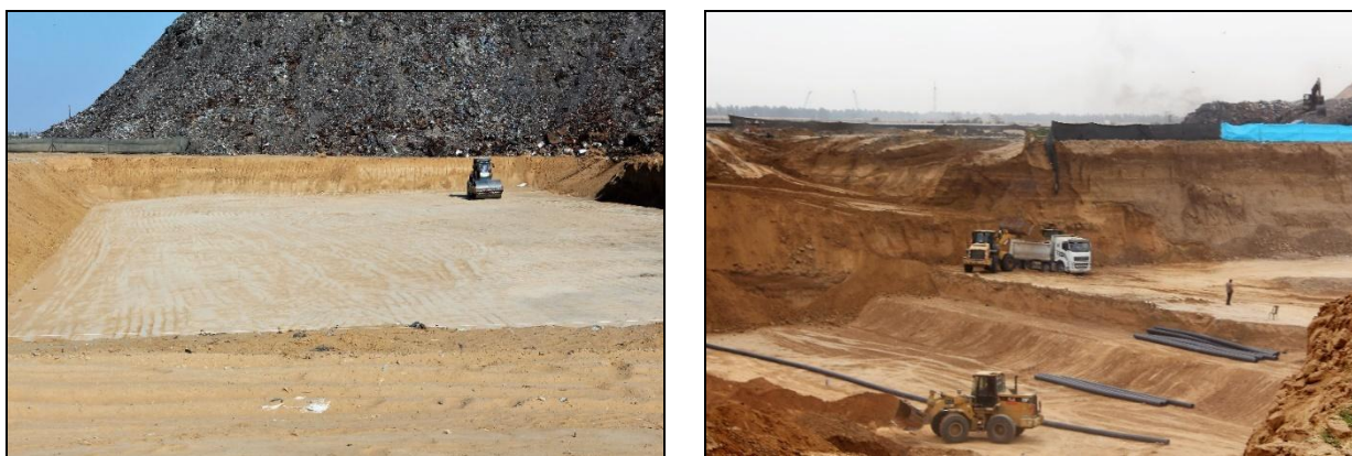
Photo 7. Photos of the excavation work in the new landfill in Al-Fukhary area during 2017
